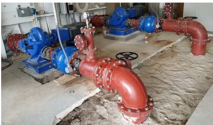
Pictured: Two of the new North Water Treatment Plant High Service Pumps
