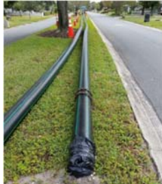
Pictured: Fused HDPE pipe laid out for the Wilshire Force Main Replacement.
