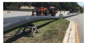
Pictured: Fused HDPE pipe ready to be drilled for the Seminola Force Main Replacement.
